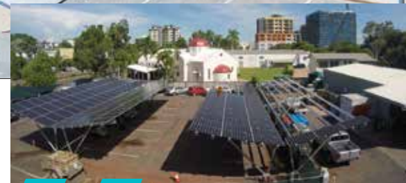
Coleman's Printing Solar Carpark 60 kW, alongside a 40 kW rooftop system
